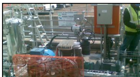
ES15 (15m 3 /h) Oily Water Separator
