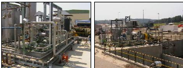
Spill Recovery System and 20m 3 /h Engineered Oily Water Separator solution at Pump station
