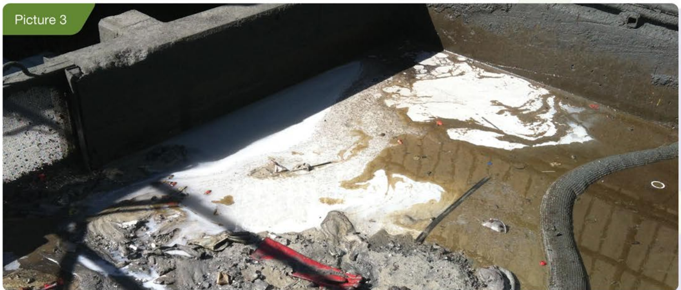
Trash & debris in oily water collection pit.
