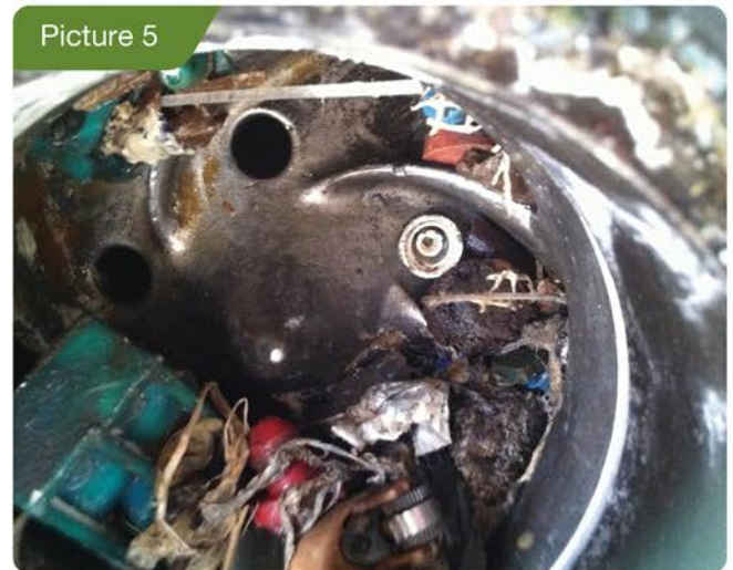
Worn and damaged pump impeller. Caused by debris.
