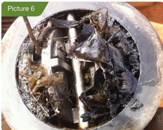
Check valve blocked by oily water debris.
