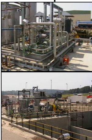
Spill Recovery System and 20m 3 /h Engineered Oily Water Separator solution at Pump station
